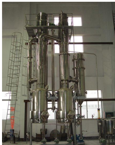
Plate 1. Falling Film Vacuum Evaporator
